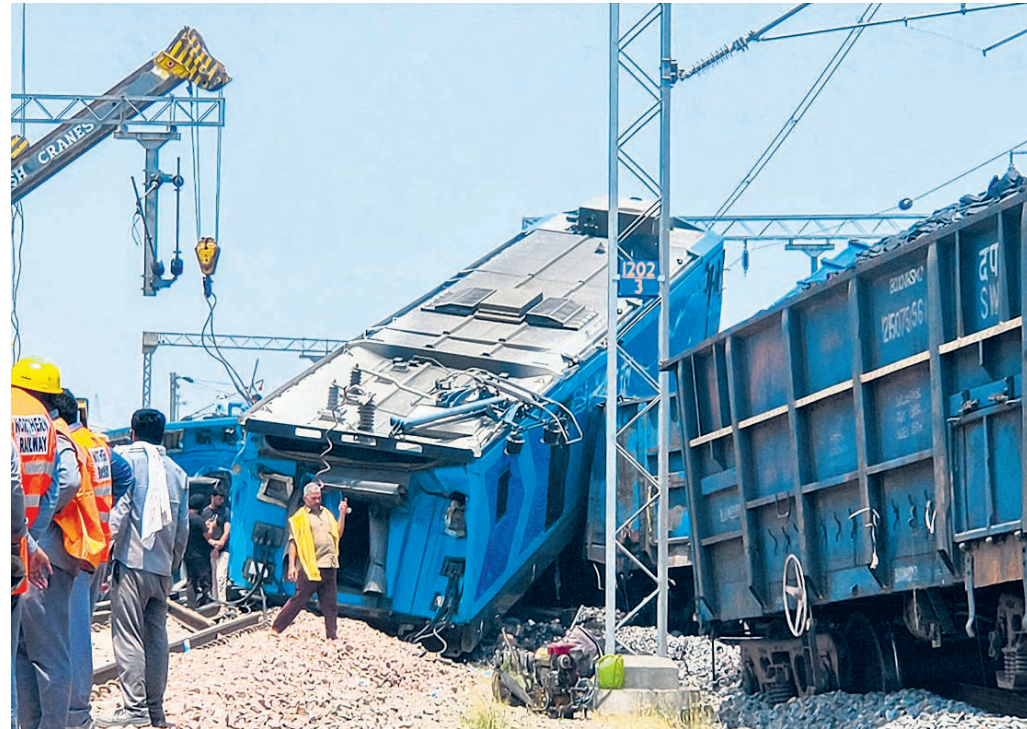
Restoration and relief work underway after a goods train derailed in an accident at Sirhind in Fatehgarh Sahib
