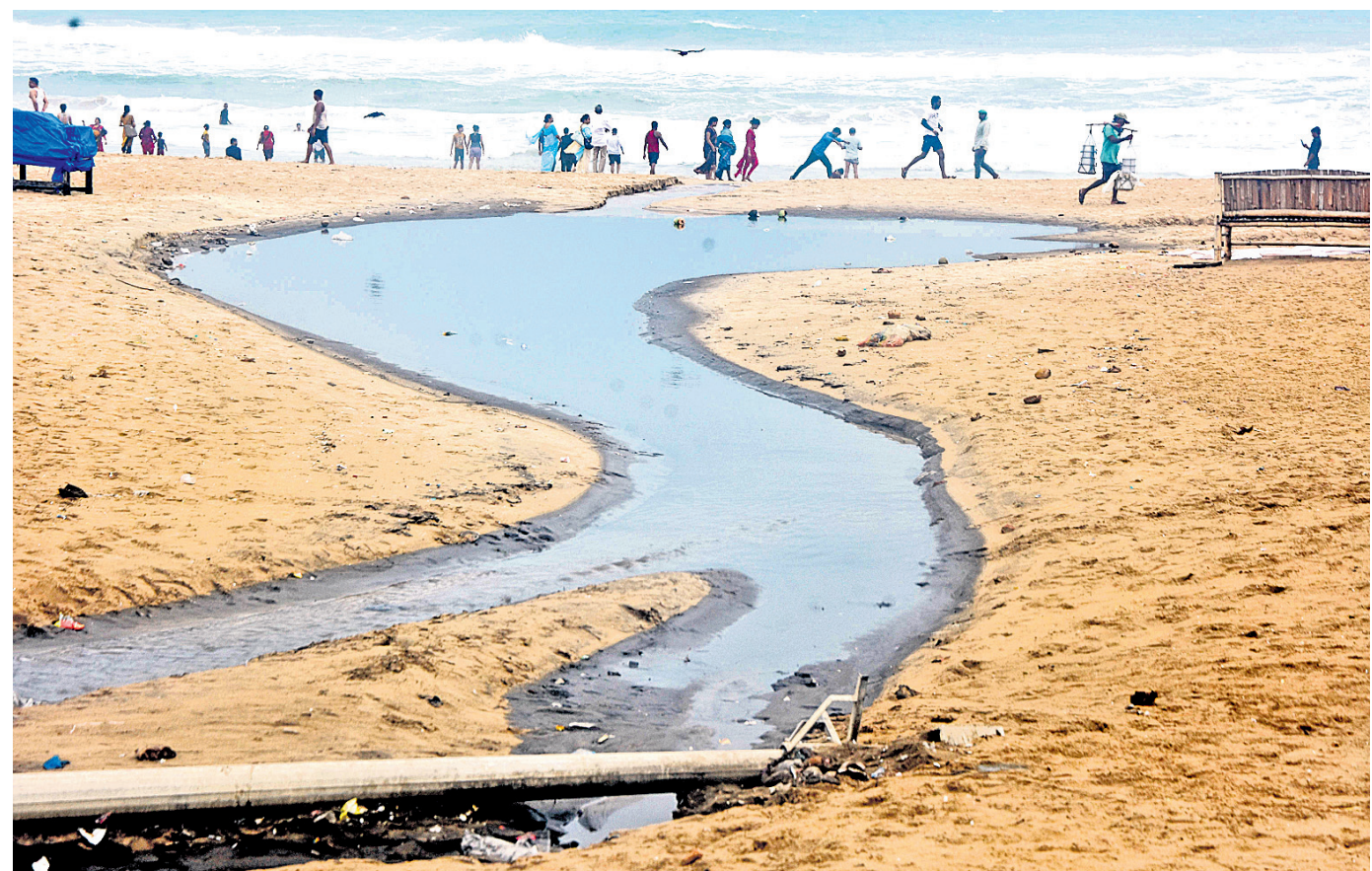
BEACH BEAUTY TURNS BLEAK: Hotels release untreated sewage water into the sea along with solid waste near Chaitanya Chowk in Puri, Saturday
