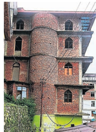
The Shimla Municipal Commissioner's court had October 5 ordered demolition of the three unauthorised storeys of the five-storey mosque
