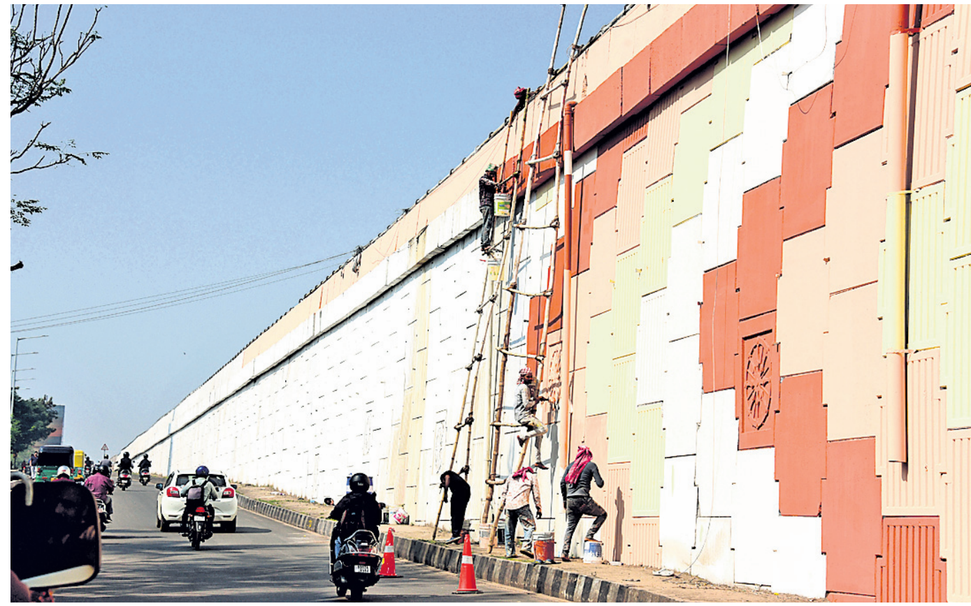
SPRUNGING UP: Workers engage in beautification work of the Rasulagrh overbridge in Bhubaneswar, Saturday ahead of Pravasi Bharatiya Divas in January 2025
