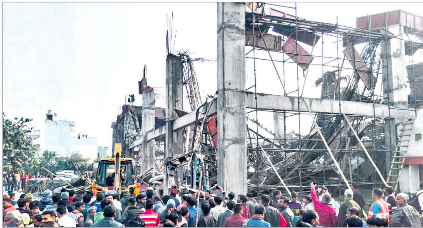
SALVAGE ACT: Rescue operation underway after an under-construction building collapsed at Kannauj railway station in Uttar Pradesh, trapping two dozen workers under the rubble, Saturday. At least 23 people have been injured in the incident. Six of them were pulled out of the debris and rushed to a hospital. PTI PHOTO
